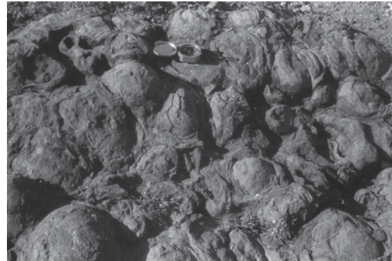
Fig.6.4 : Exfoliation (Flacking) and granular disintegration
